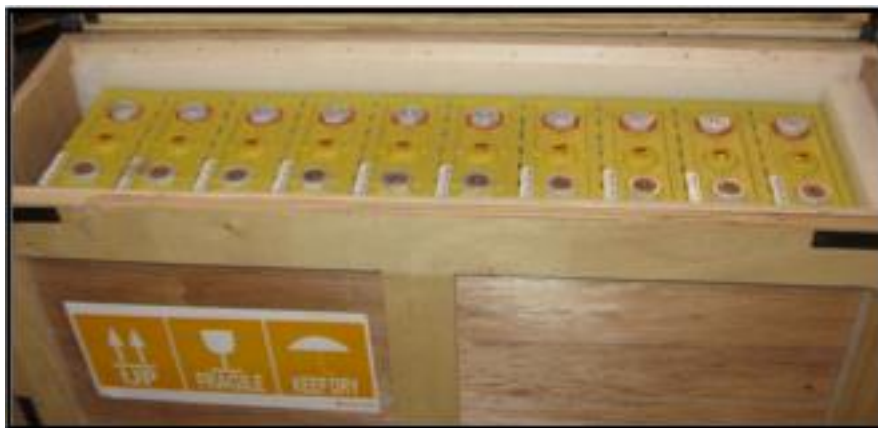
Figure 3: Photograph of lithium/iron batteries
